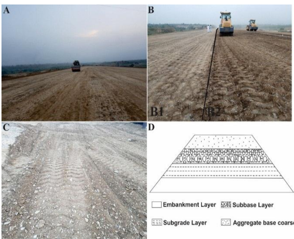
Fig. 2 (A) Showing the compacted embankment layer. (B) The glance of subgrade while (B1) compacted subgrade layer (B2) until not compacted. (C) Showing subbase layer until not compacted of project E-35 Phase-I (D) Showing embankment, subgrade, subbase, and aggregate base coarse of highways.
