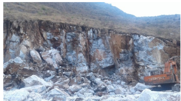
Fig. 5 A marble mining quarry of Sunny Grey Marble of Bampokha District Buner.
